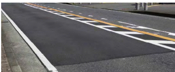
Section of public road surfaced with the new material for tests (the part of the darker color)
